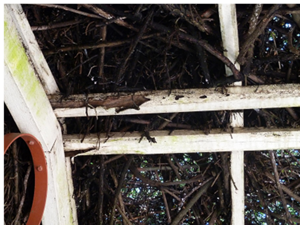
Rotting timber in Pergola near entry gate
