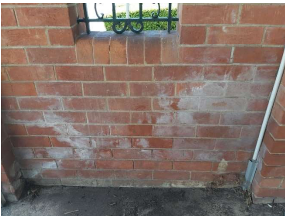
a. Rising damp on entry gate brickwork
