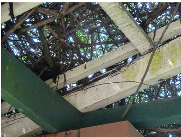
Rotting timber in Pergola near WWI memorial
