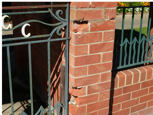
b. Damaged brickwork on entry gate
