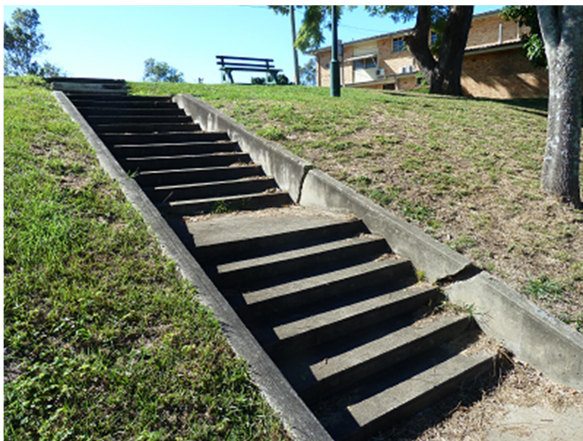
Concrete stairs showing cracking in side wall
